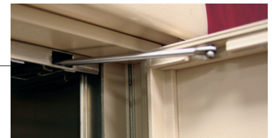
Stainless steel hold open door catch on each side of master gate
